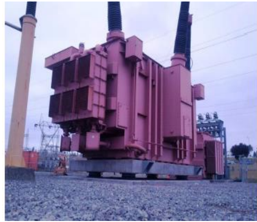
Figure 1. The seismically isolated transformer in Vancouver
