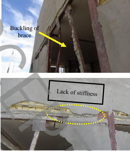
Fig. 2. (Top) buckling of brace in out-of-plan, (Bottom) lack of stiffness in link beam (Authors)
