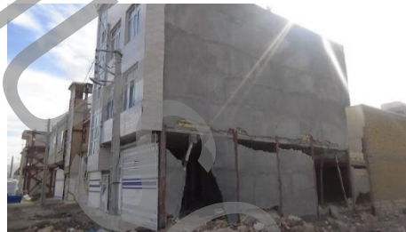
Fig. 1. Damaged three-story building with EBF system in the Sarpol-e Zahab earthquake (Authors)
