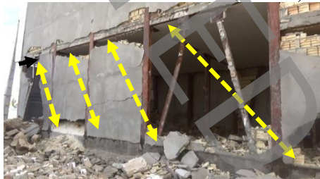
Fig. 3. Tolerate part of the lateral load by formation of the compression diagonal struts of infill walls (Authors)
