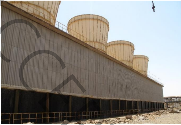
Figure 2. General view of the studied cooling tower
