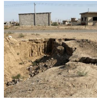
Figure 1: Image of the research site in the Dashli-Brun area (adjacent damage)
