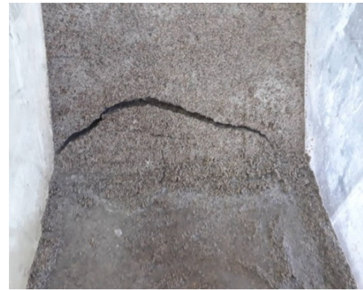
Fig. 3. Failure shape with 5% nano-lime covering
