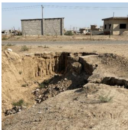
Fig. 1. Image of the research site in the Dashli-Brun area (adjacent damage).
