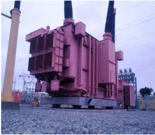
Fig. 1. The seismically isolated transformer in Vancouver
