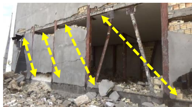
Fig. 3. Tolerate part of the lateral load by the formation of the compression diagonal struts of infill walls (Authors)
