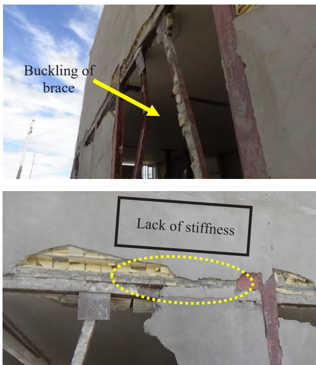
Fig. 2. (Top) buckling of brace in out-of-plane, (Bottom) lack of stiffness in link beam (Authors)
