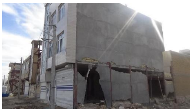
Fig. 1. Damaged three-story building with EBF system in the Sarpol-e Zahab earthquake (Authors)
